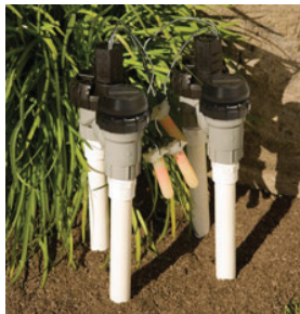
Irrigation System Atmospheric Vacuum Breaker
